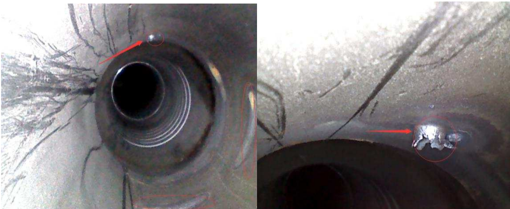
The inside flaw of the exhaust pipe
